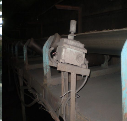
Belt sway switch
