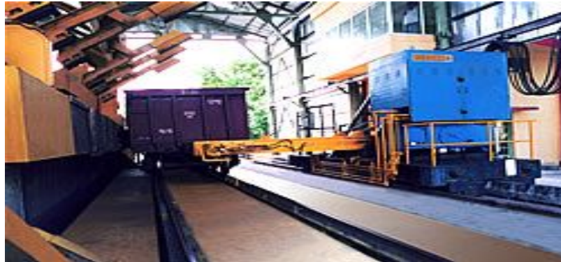
Side Arm Charger for hauling rake of wagons, placement of wagons on tippler table and evacuation of empty wagons from tippler table.
